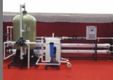
DigiLite Industrial RO Plant
