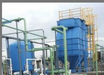
Klarimax Sewage Treat Plant
