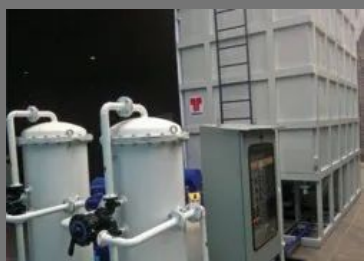
Sewage Treatment Plants
