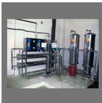
Packaged Drinking Water Plant
