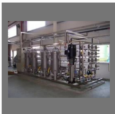
Packaged Drinking Water Plant
