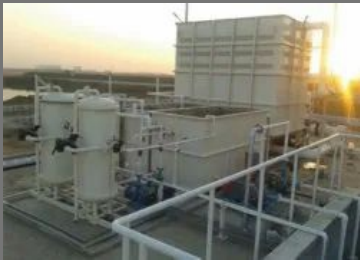
Biofiltration Sewage Treatment Plant
