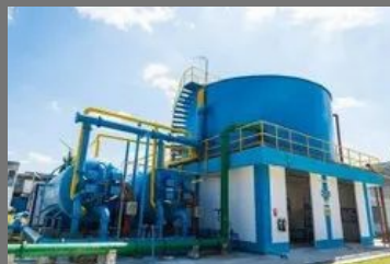
Fully Automatic Industrial Water Treatment Plant
