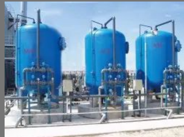
Water Distillery Water Treatment Plant
