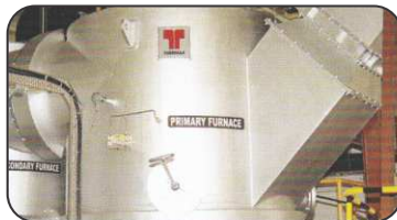
Incinerator | Infections & hazardous waste treatment
