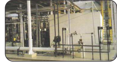
Seqtreat - Sequential Batch Reactor Technology | 100 KLD & Above
