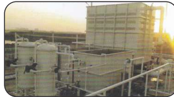
Biofilter | Low sludge sewage treatment plant
